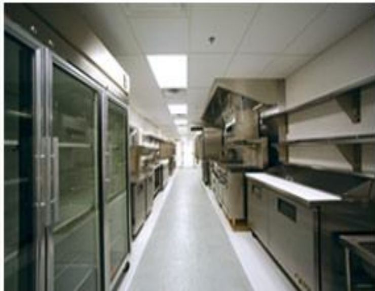
Through Polar Leasing Company partners, complete temporary kitchen and base camp setup is available
