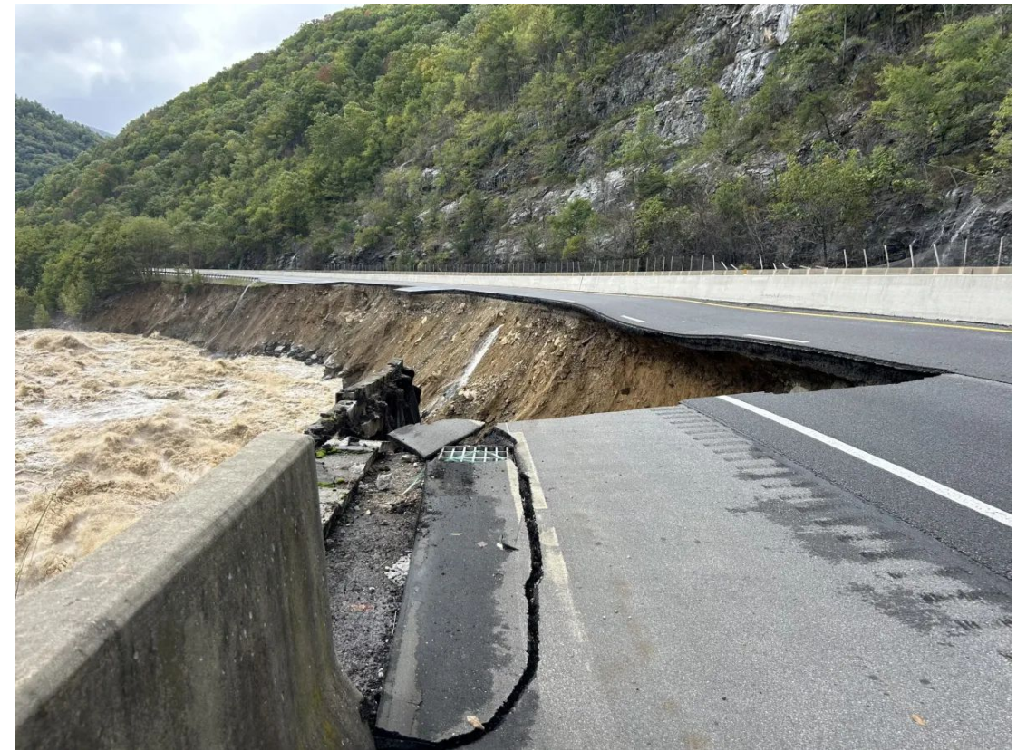
NC/TN State Line I-40 Hurricane Helene
